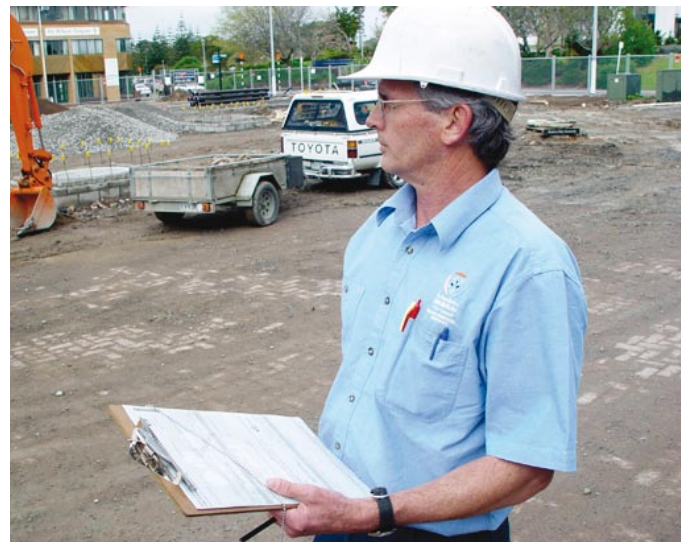
Peter Moloney , team leader building compliance with Manukau Building Consultants, doing a site inspection.
